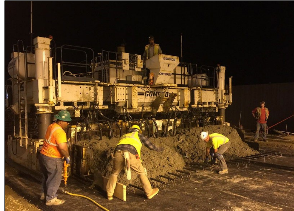
Paving, signing and striping using rollers, concrete trucks, delivery trucks, dump trucks, loaders, street sweepers, sign and stripe trucks.
