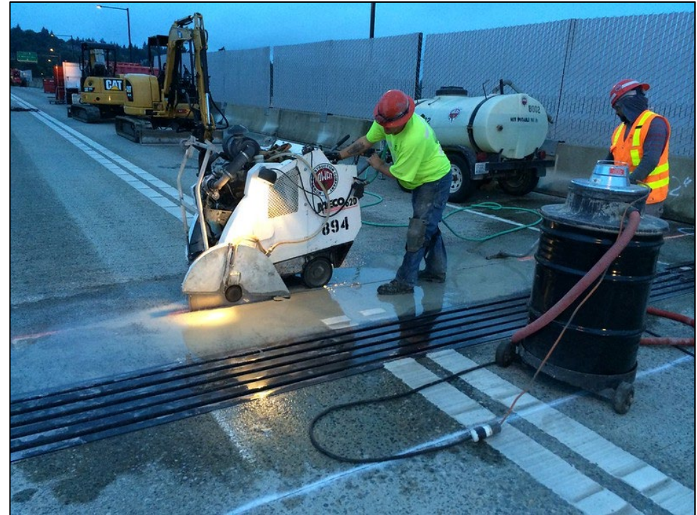
Concrete sawing with equipment including compressors, dump trucks, loaders, debris trucks and street sweepers.
