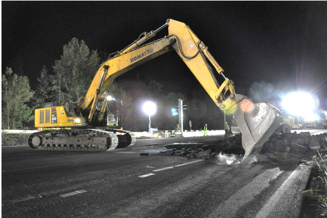
Excavations for digging, trenching, embankment and paving using equipment including dozers, excavators, vibratory rollers and drill rigs.
