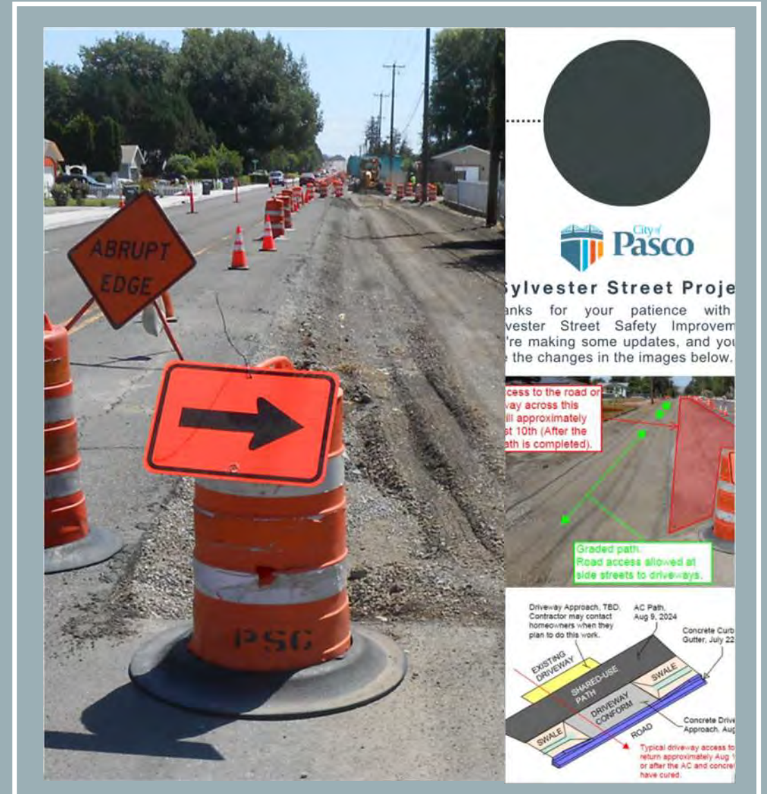
Reference Image (Left): Phase 2 near Rd 39 and Sylvester St Reference Image (Right): Door Hanger
