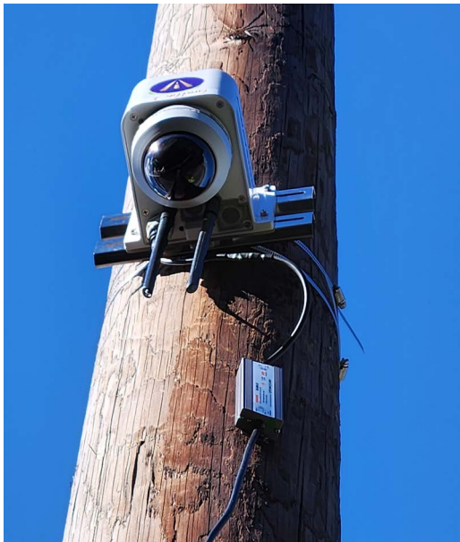
Figure 8a. AIWaysion device installed
