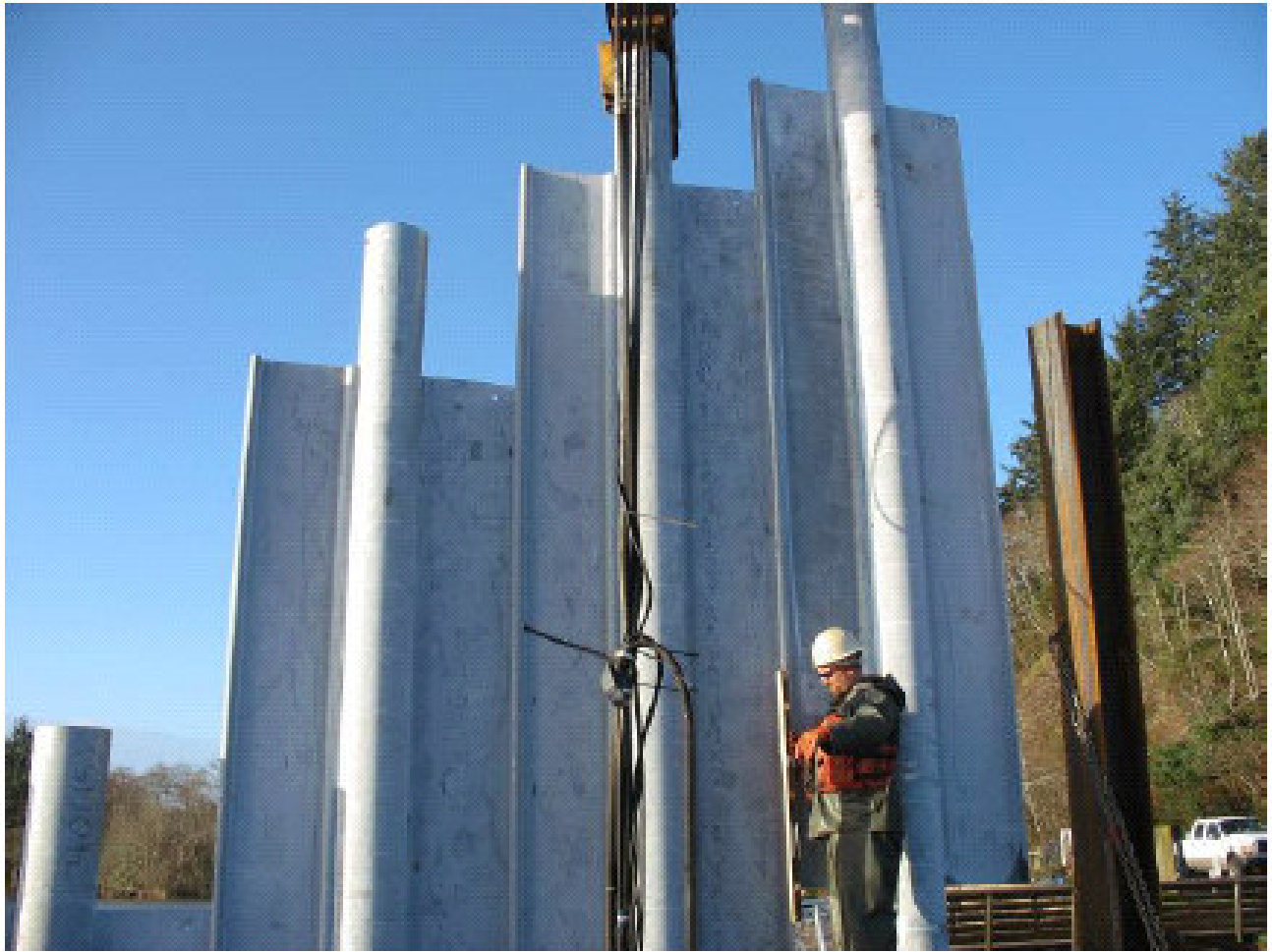
Figure 2: 12-inch diameter steel piles with interlocking ‘wings’ used to create the wave barrier (photo courtesy of Washington State Parks and Recreation, R. Johnson).
